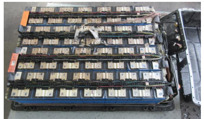
Figure. 10 Inside View of DUT
